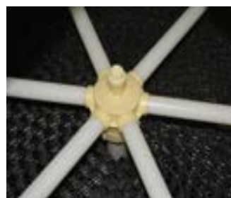
Cooling Tower Distribution Pipe
